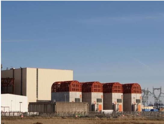
3-MWe station blackout diesel generators [DUS]
