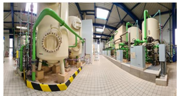
Dampierre-en-Burly NPP demineralisation station © EDF
